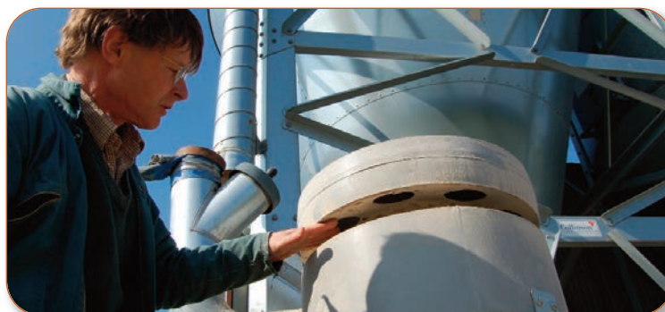
The cyclone attaches to the exhaust pipe on feed bins to collect dust
